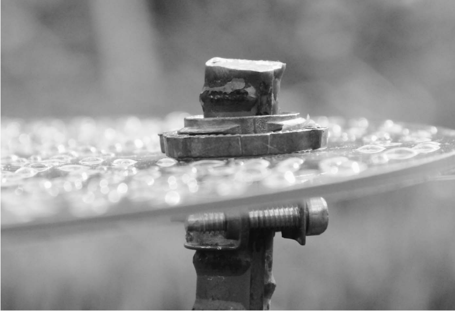
Fig. 5. Detail of cable clamp holding polycarbonate cover to rebar support.
